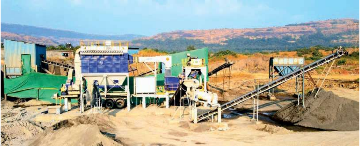
The first Wheel-Mounted Mobile Dry Sand Air Classifier Plant at a project site near Pune
