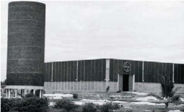
L&T's Bangalore Plant under construction which went on to become L&T-Komatsu Limited
